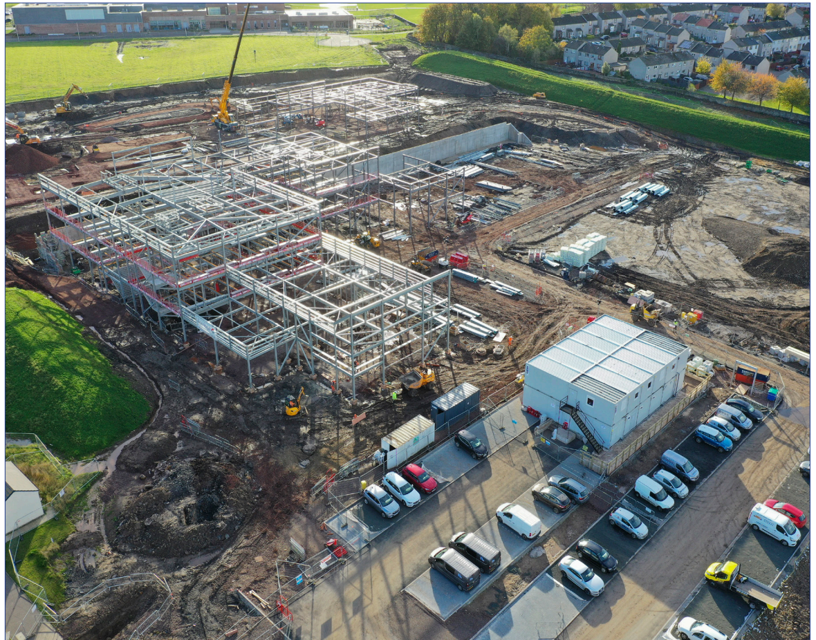
Wallyford Learning Campus – The first LEIP funded school to progress on site
